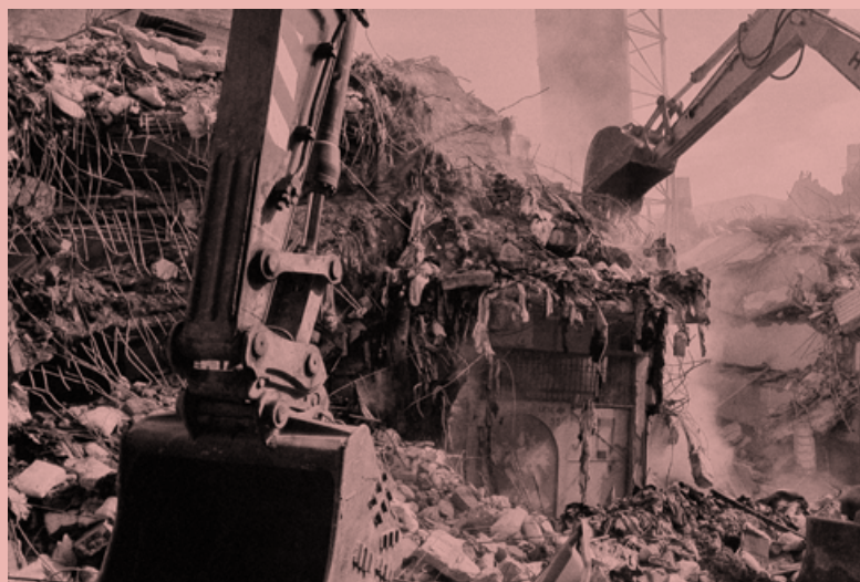
The burned-out textile factory was demolished, but the questions raised by this disaster can no longer be erased from the world. ©HBWWF (Home-Based Women Worker's Federation)
